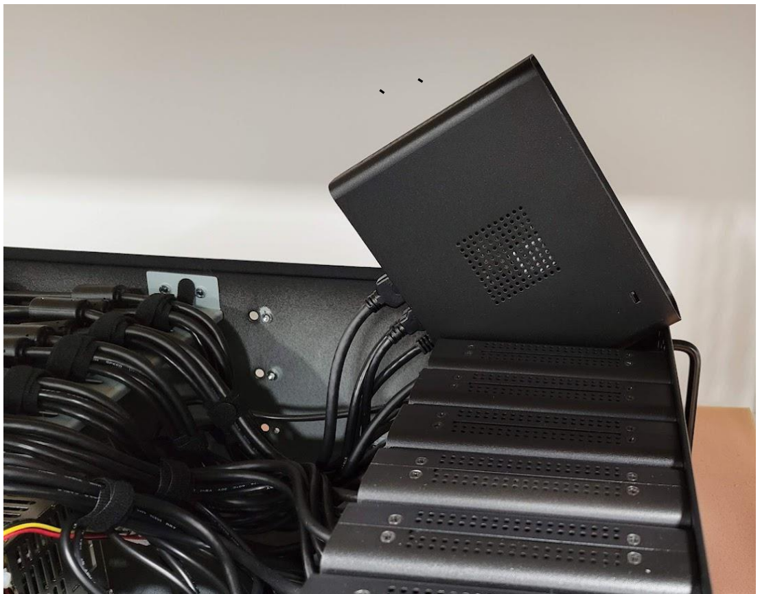
Figure 8 Cabling units outside of drawer
