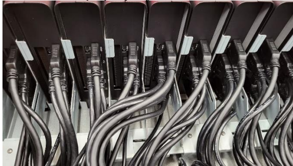
Figure 13 ClearCube devices installed in unit
